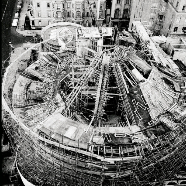
Construction of the main rotunda, ca. 1958. Photograph by William H. Short © The Solomon R. Guggenheim Foundation, New York.
